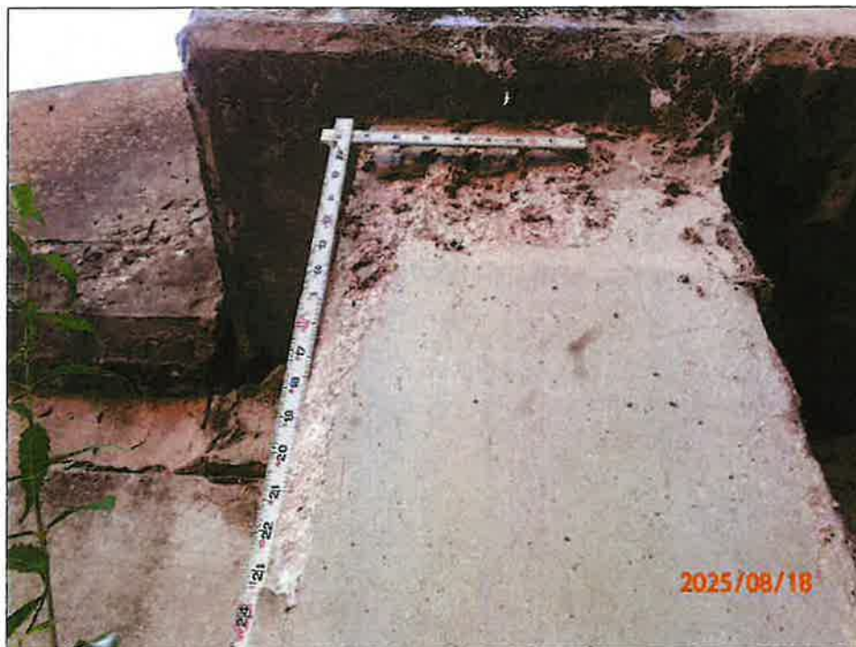
Photo 20 – Spall at Pile 2-1, 2-2 and 2-3, northwest corner.
