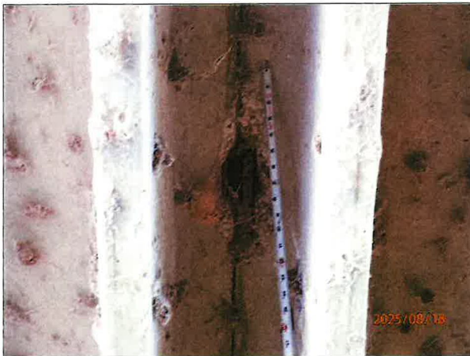
Photo 8 – Spalls at the joint between the beams at the top flange.
