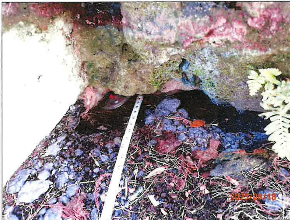
Photo 36 – Area of previous repair and erosion at the southeast seawall.
