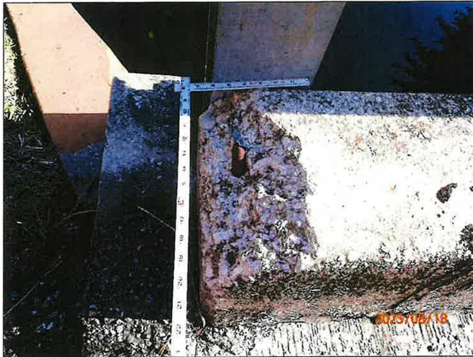
Photo 7 – Spall at the north curb, west end.
