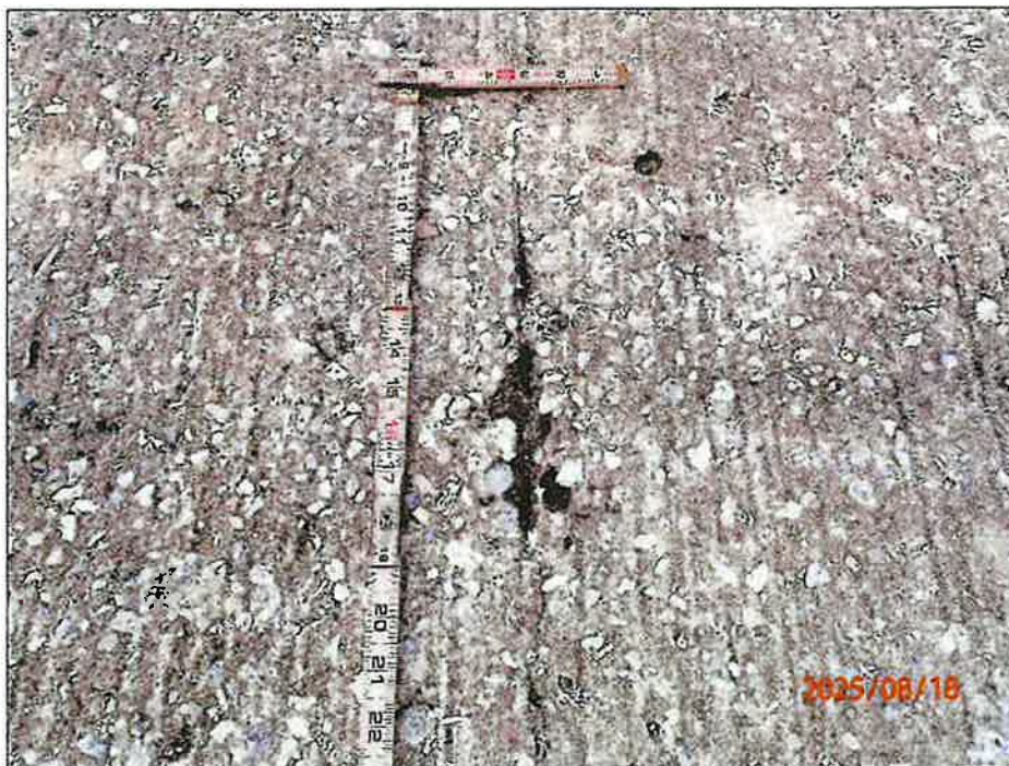
Photo 6 – Longitudinal and transverse cracks on the deck top.
