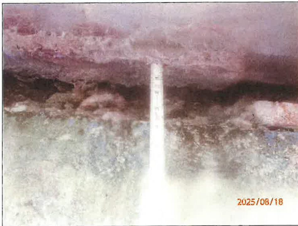
Photo 16 – Settlement at the abutment backwalls.
