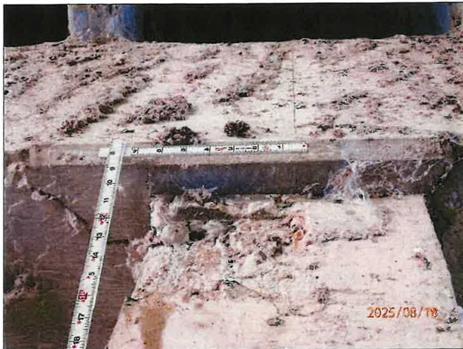
Photo 15 – Spalls/delaminations at the abutment caps adjacent to the piles.
