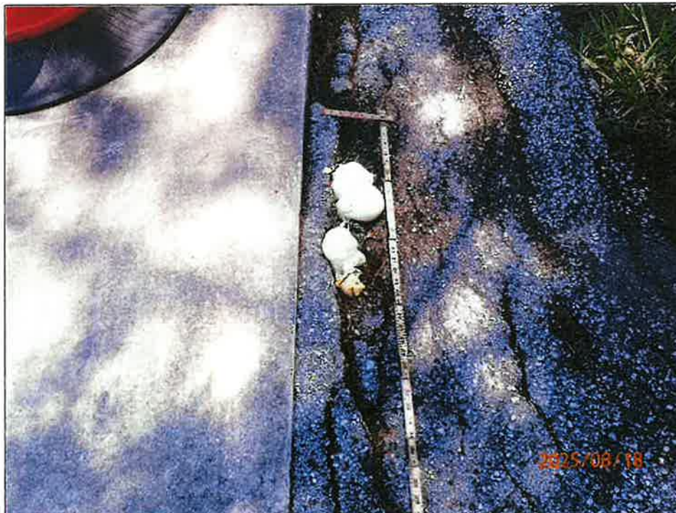
Photo 10 – East approach slab has areas of spray foam repair along the north and south edges.
