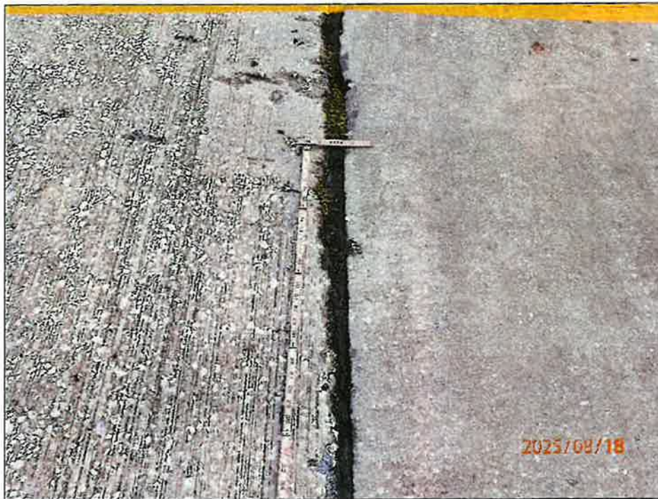
Photo 9 – Deteriorated bridge joints with some areas of missing sealant.
