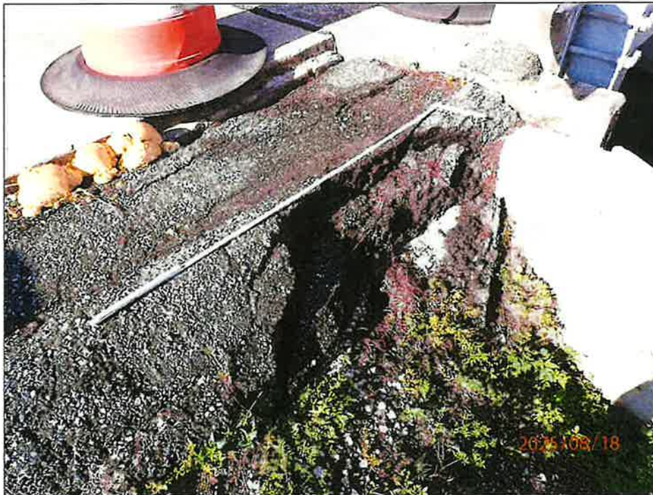
Photo 14 – Area of erosion/settlement at the east approach slab, north shoulder.
