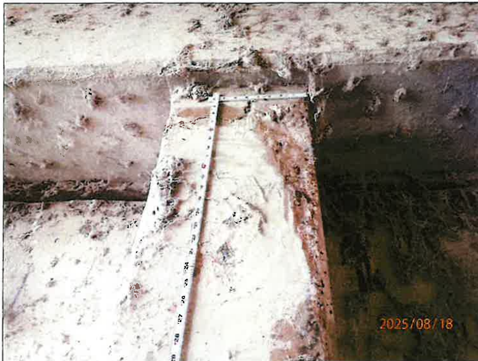
Photo 19 – Spall/delamination at Pile 1-4, northeast corner.
