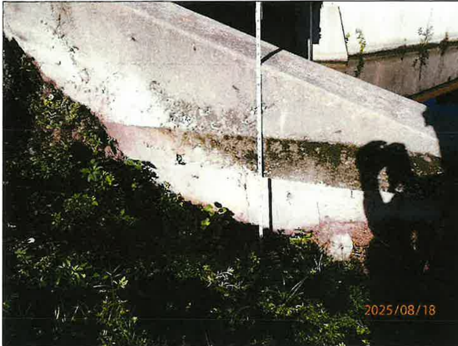
Photo 29 – Erosion hole behind northeast seawall near shoulder of bridge.
