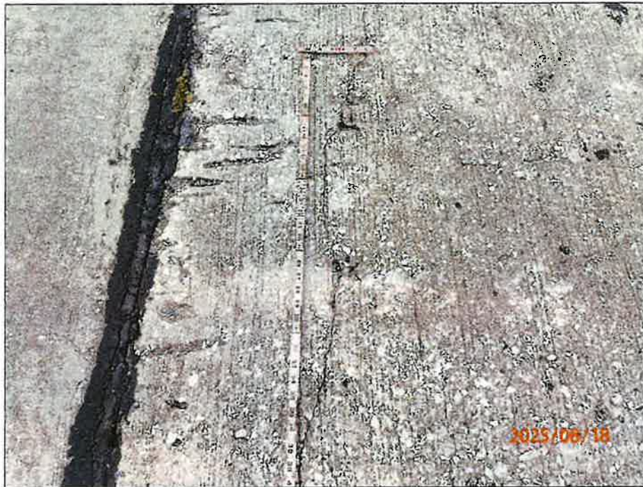
Photo 5 – Transverse crack on the deck top at both abutments.
