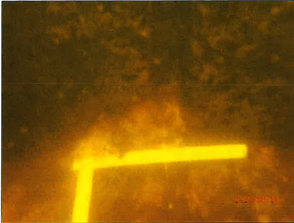
Photo 25 – Void at the northeast seawall, 3 rd panel from abutment and 1 st angle break.
