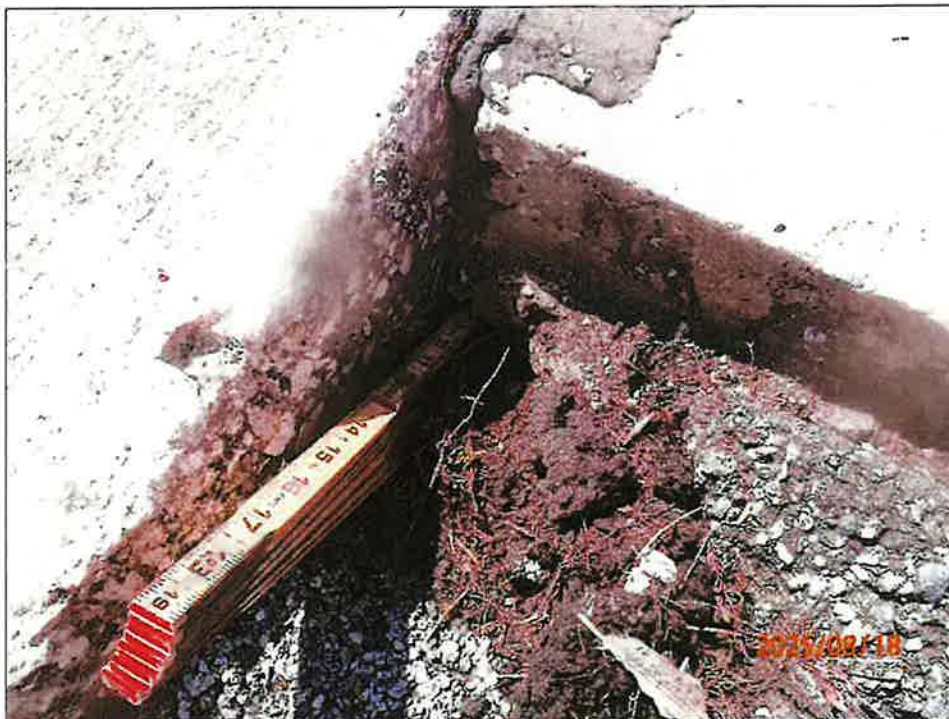
Photo 12 – Area of erosion at the west approach slab, northeast corner.
