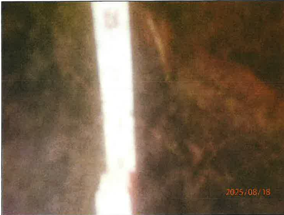
Photo 33 – Tree roots growing between seawall joints at the southeast seawall.
