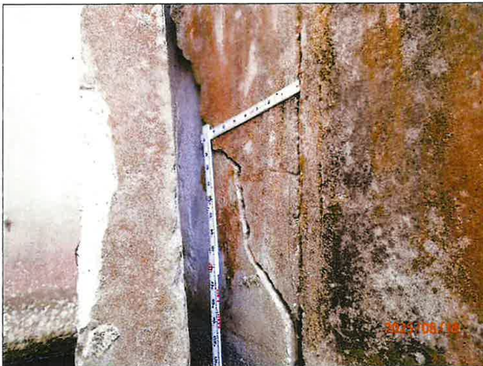
Photo 32 – Diagonal fracture at the southeast seawall, 1 st panel from abutment.
