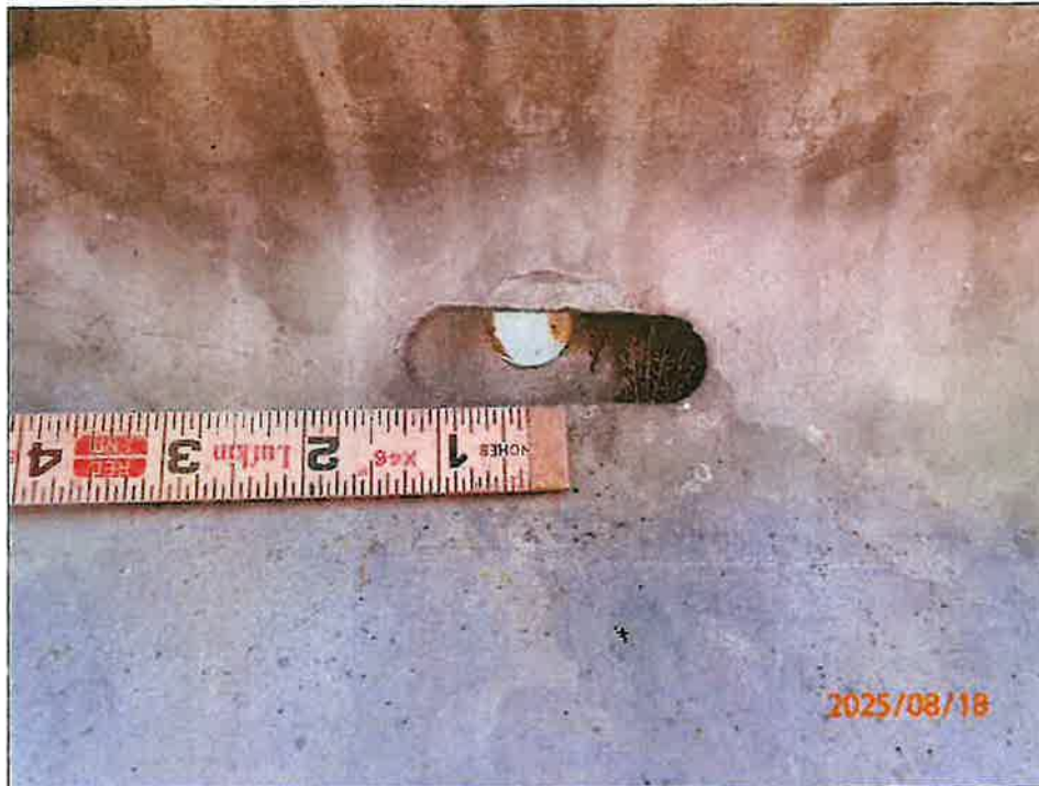
Photo 21 – Missing guardrail bolt at south bridge rail, middle post.
