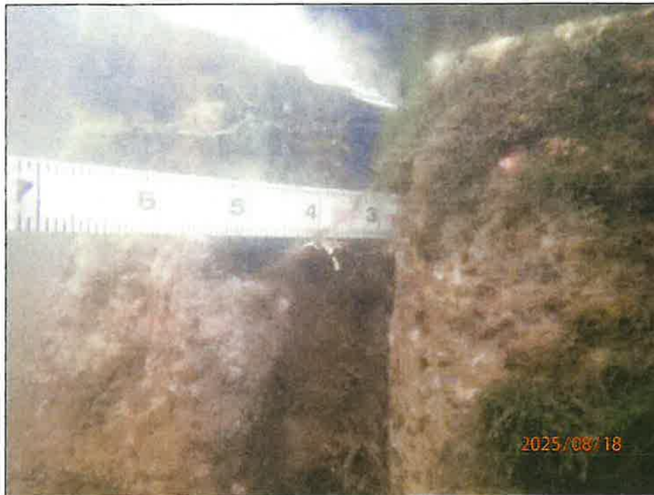
Photo 37 – Open joint exposing backfill at the southeast seawall angle break.
