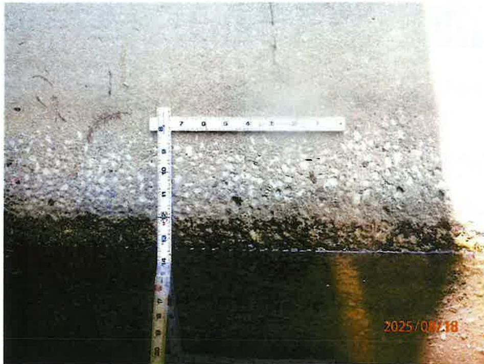
Photo 17 – Areas of abrasion at the abutment backwalls.
