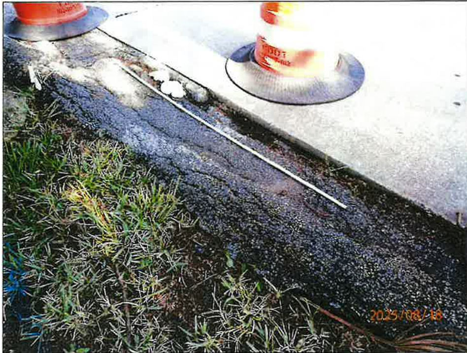
Photo 13 – Asphalt shoulder asphalt extension adjacent to the approach slab is lower in elevation.
