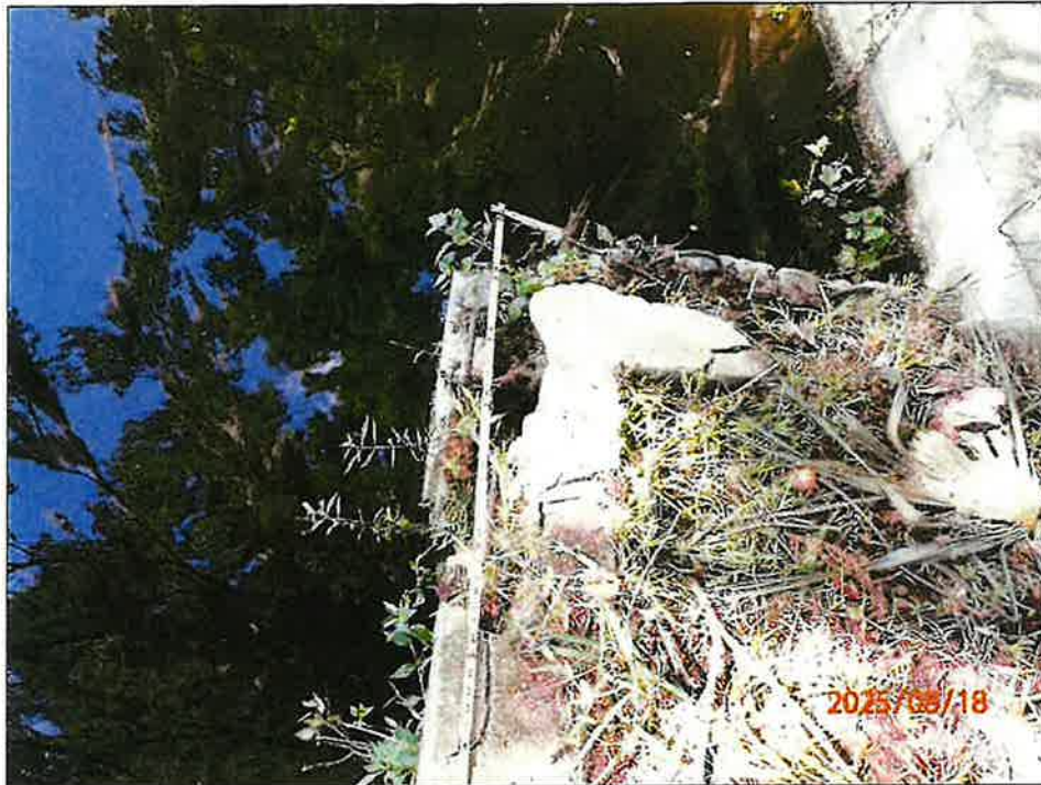
Photo 23 – Settlement at the southwest seawall, first angle break.
