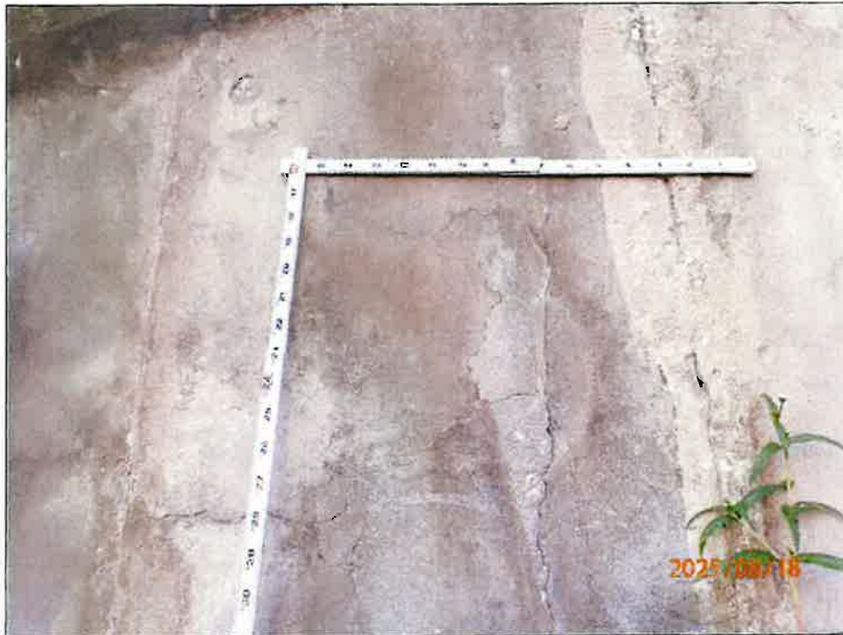
Photo 35 – Vertical cracks and associated delaminations at northeast seawall, 3 rd , 5 th , 6 th , 7 th and 8 th panels from abutment.
