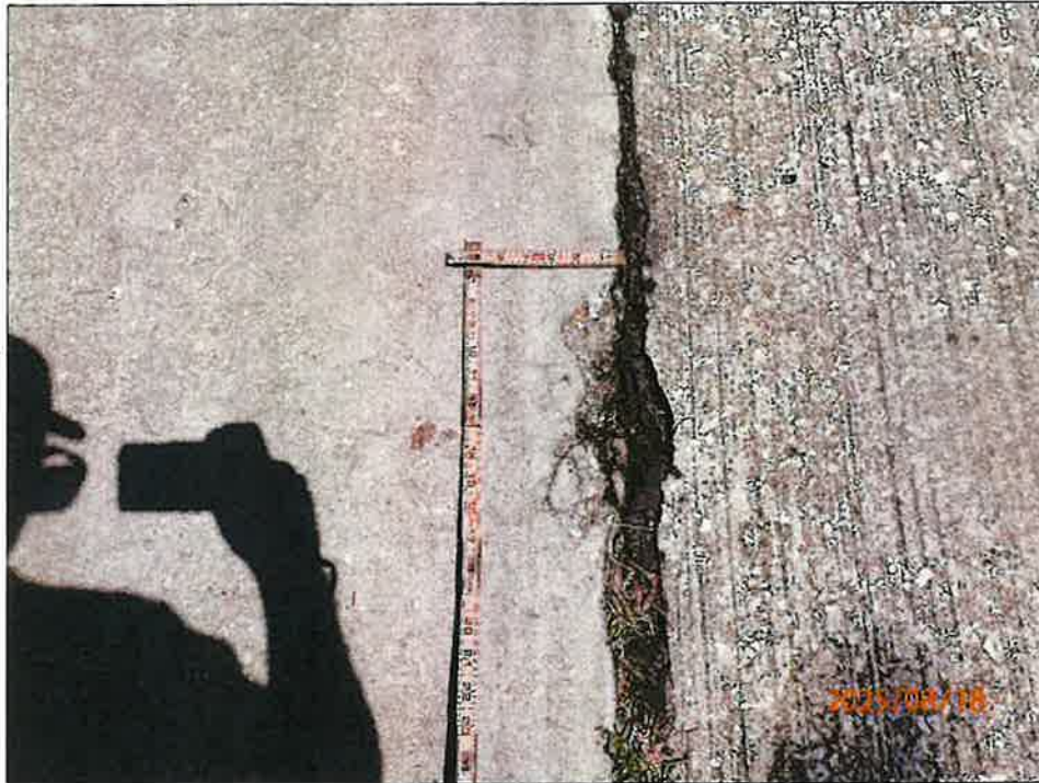
Photo 11 – Spall at center of EB travel lane, west approach slab.
