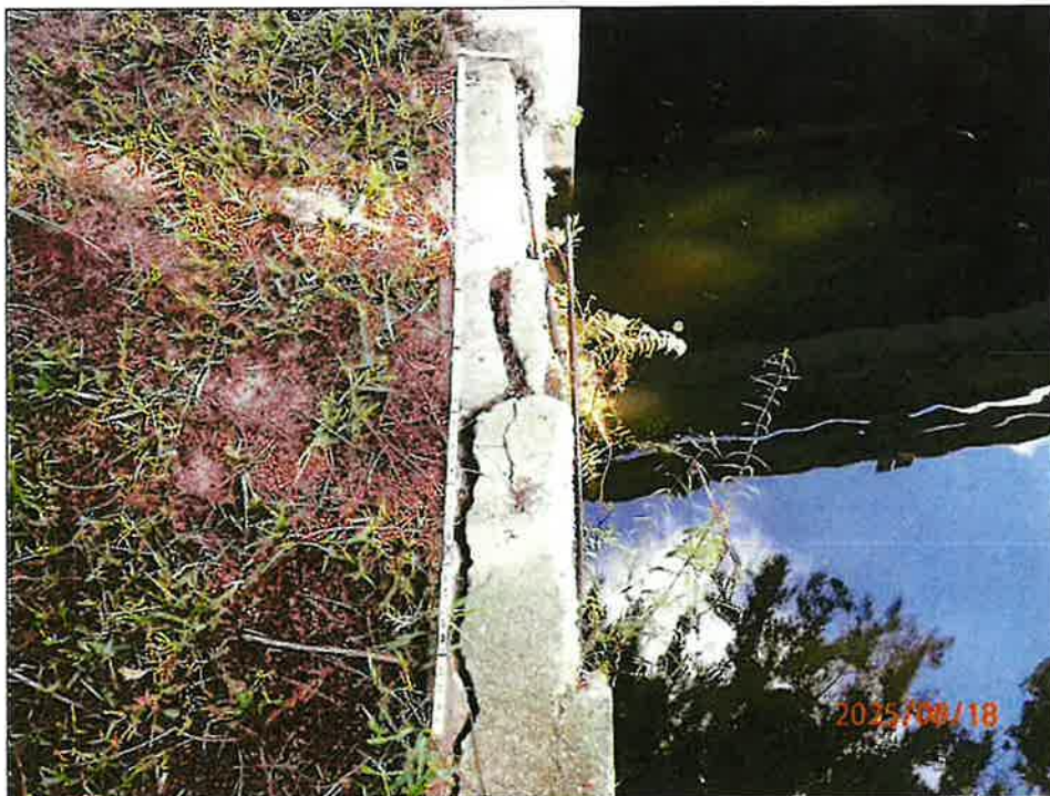
Photo 22 – Settlement at the southwest seawall.
