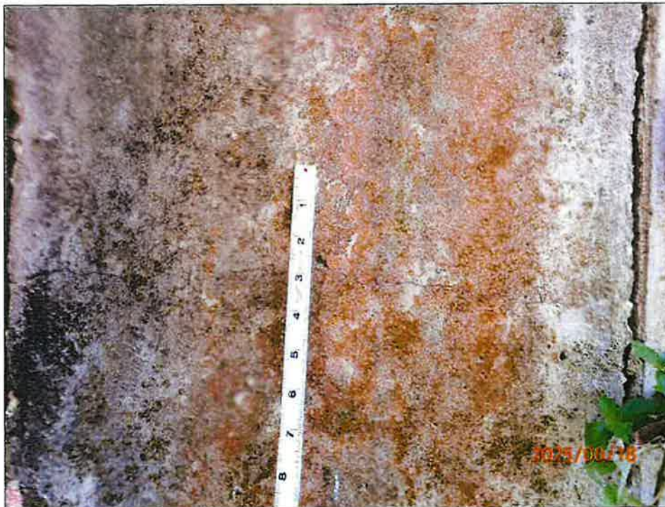
Photo 34 – Horizontal cracks on multiple panels on seawalls adjacent to the bridge.
