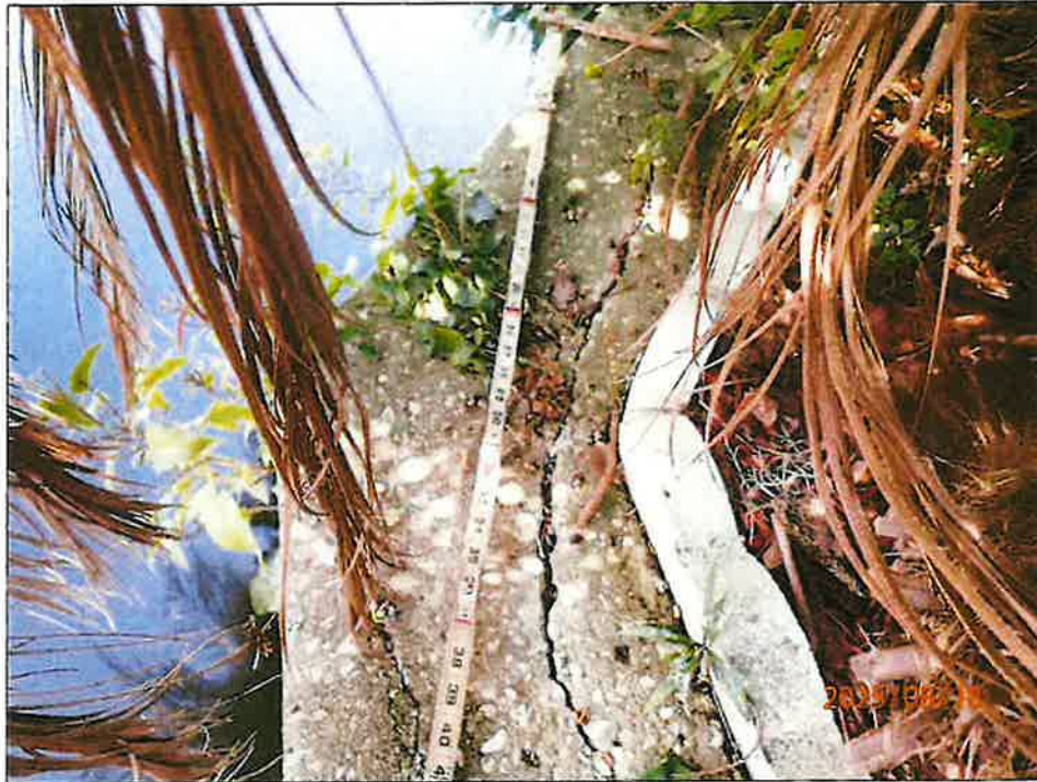
Photo 31 – Longitudinal cracks at the northeast seawall cap, top face.
